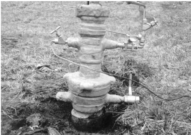
#2A Wax-Tape (aluminum pigmented) easily applied to a difficult-to-protect wellhead. Note the complete conformity to the irregular surfaces.
