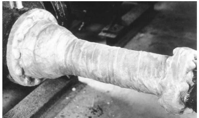
Sweating meter run pipe protected with #2A Wax-Tape.
