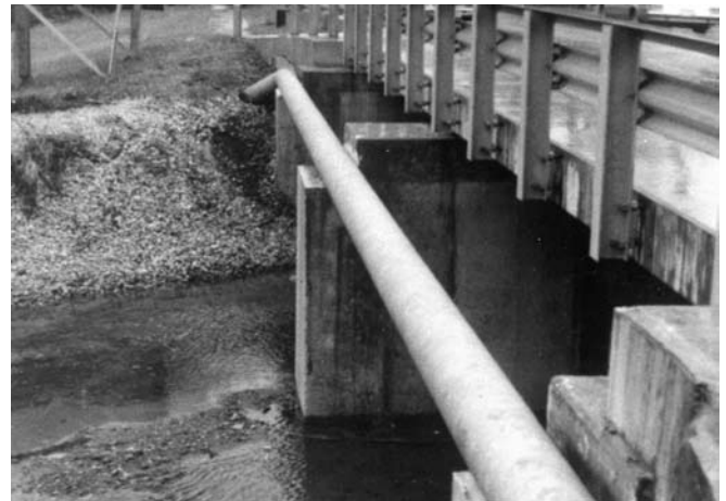
#2A Wax-Tape applied to bridge span, providing corrosion protection from road salt, physical damage and atmospheric corrosion.
